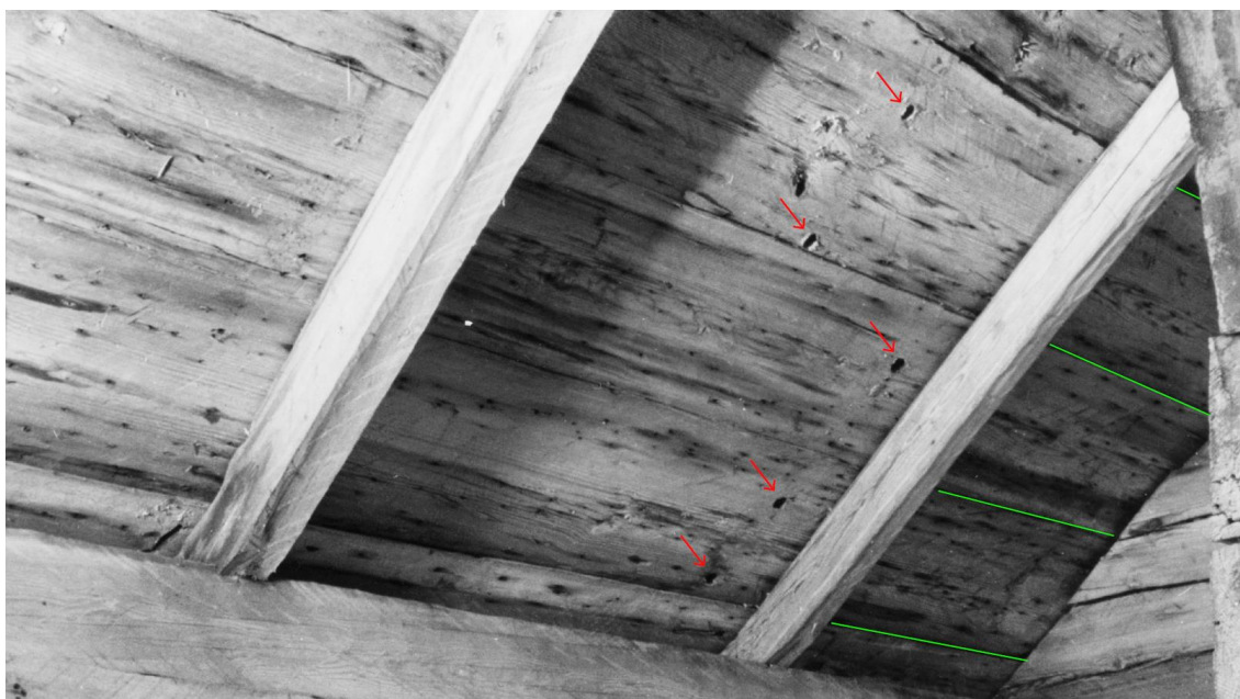
Fig. 8. Roofing and trefoil boards from the Södra Råda church. The photo shows the roofing boards of the sacristy of Södra Råda. At first glance, they seem to be original since it is clear that the sprätthuggning technique has been used. Closer examination makes it possible to see that they most probably are original but displaced. The red arrows point at holes where nails or pegs were used to fasten the boards to a rafter. The green lines illustrate the width of the boards. From the picture, the width of the boards can be determined to be around 35 centimetres. Photo National Heritage Board, ATA.
